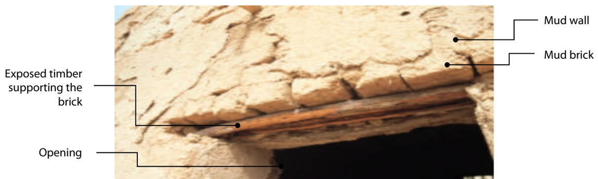
Figure 1: Lintel supported with an exposed timber
